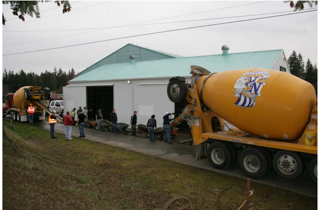
Navy personnel wheel concrete into the Pole Barn from Fred Hill Materials trucks Photo by Gary Beanland
